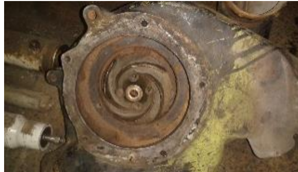
Figure 2: View from the pump's upper cover
